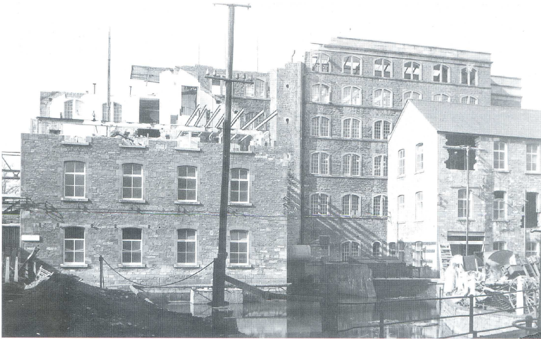
Above and Below - The Old Mill Building being demolished down to two storeys 1935.
