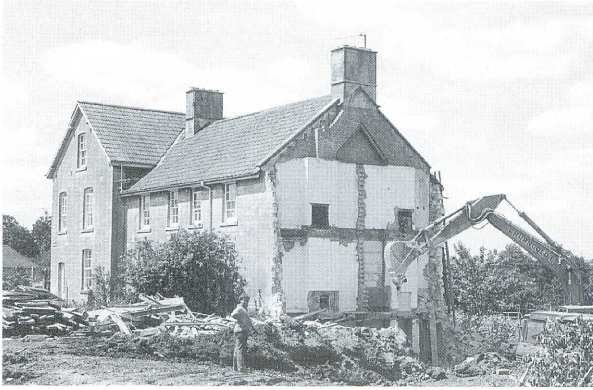
Three of the Nasmilco Cottages being demolished to make way for the Dessert Plant Expansion 1987.
