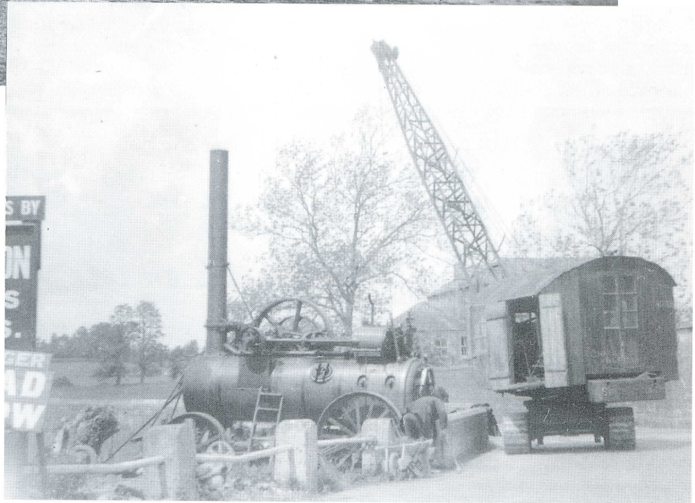
Above - The Old Mill being Demolished 1935. The New Process Block and Tinshop can be seen on the right.
