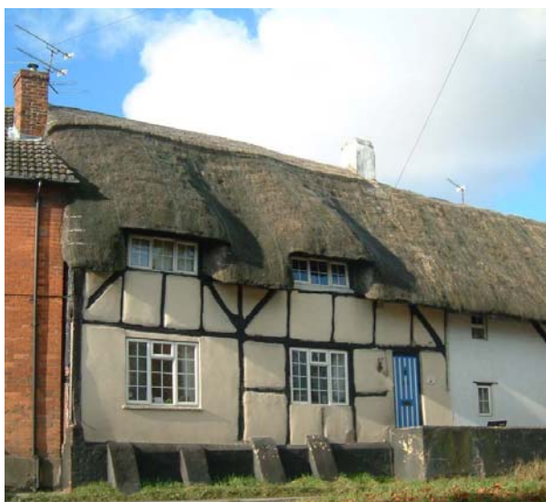
pvcU casements fitted to Listed Buildings. A poor imitation of the original - frame sections are too thick and the glazing bar sections too thin.
