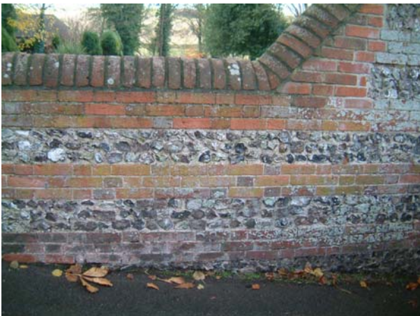
A brick and flint banded wall with half round dense clay coping bricks
