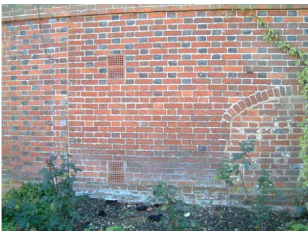
Red brick walling. Vitrified headers in Flemish bond Left - late 18 th century. Right - early 19 th century.
