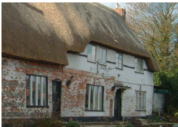
Windows of unsuitable design fitted to listed buildings. Here upper windows interrupt the timber structure and the lower fixed lights are of single sheets of glass. Removal of paint is in progress from the brick and flint walls. If the correct methods are being used this could enhance the building.
