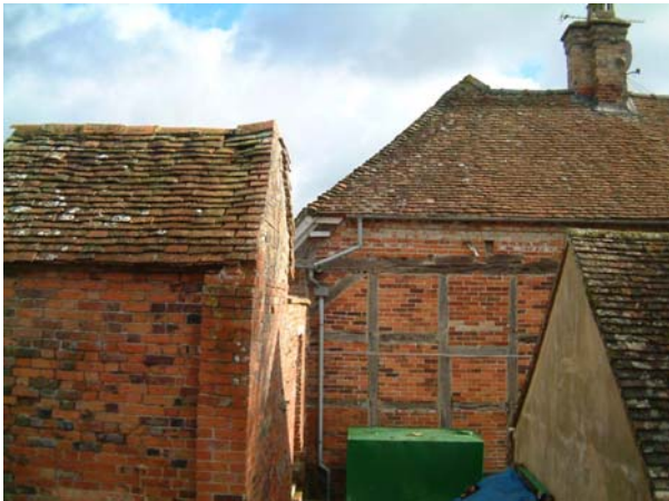
Manor Farm house. The 17 th century timber frame has been infilled in brick concurrently with extensions to the house in the 18 th century. The roofs are of handmade clay plain tiles of the 18 th and 19 th century.
